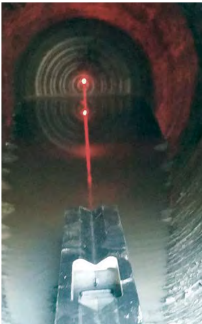
Laser guidance made sure the PDC reamer was cutting straight on grade
