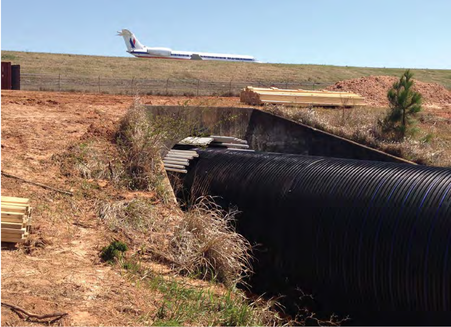
A lightweight cellular grout was used in multiple lifts through tubes at the headwall as well as grout ports in the pipe.
