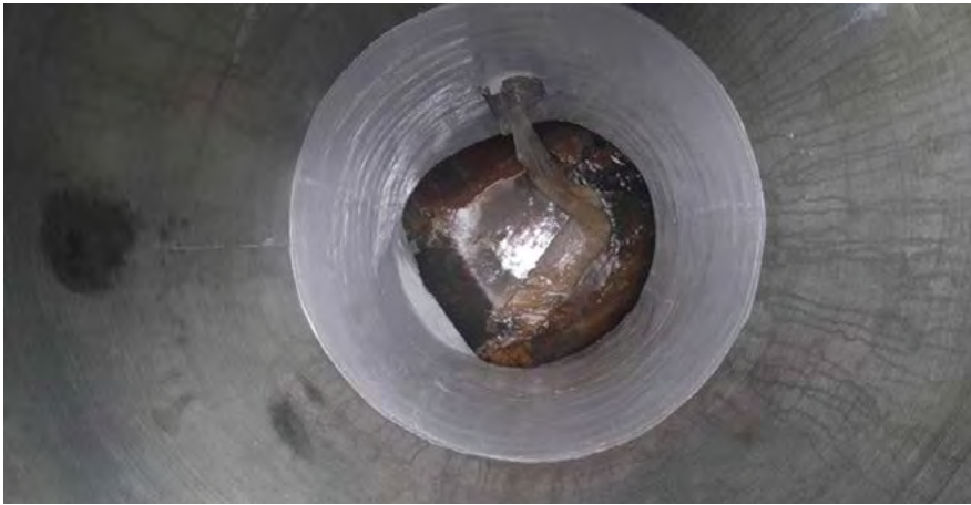
A cementitious lined manhole with bottom section epoxy lined after 54-inch CIPP was externally sealed for infiltration
