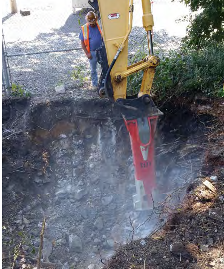
Hard limestone under railroad tracks presented obstacle to completion of natural gas pipeline project
