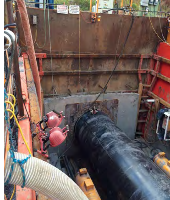
59-inch steel casing was used in lieu of 60-inch to increase overcut in self-supporting ground
