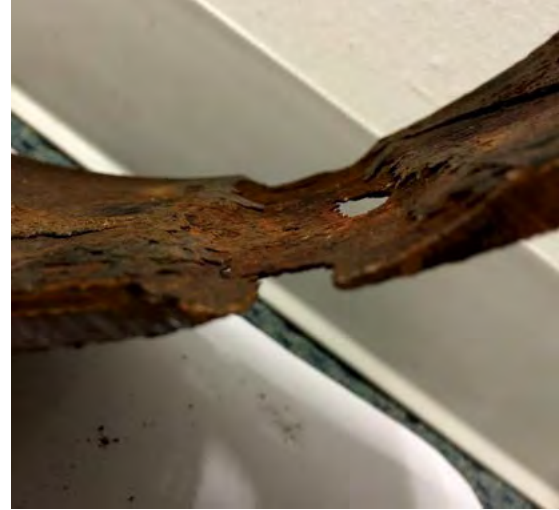
Invert of Failed Pipe Section
