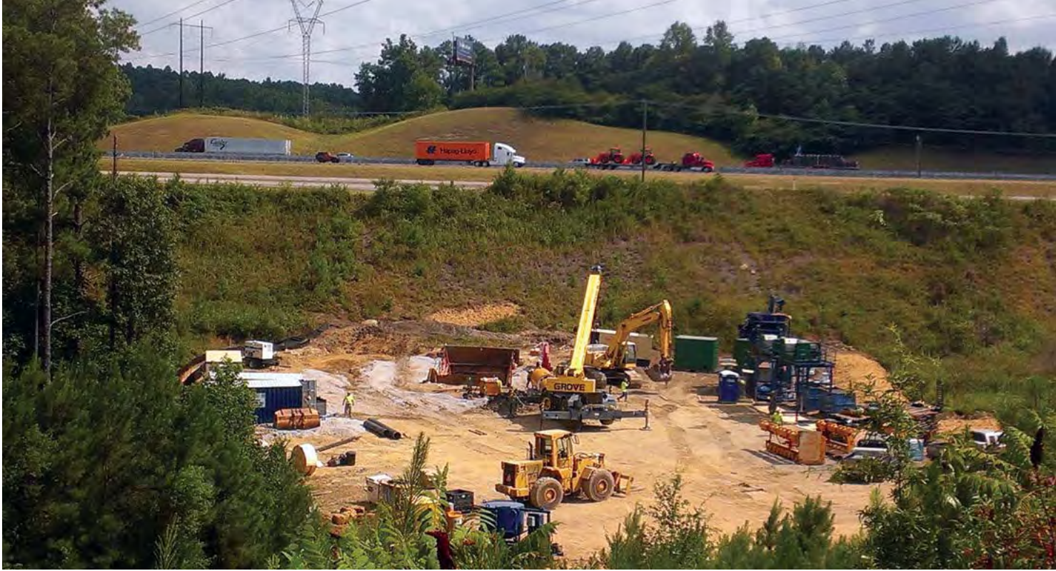
Launch shaft, under 230kv power lines, with view of Highway 78 and Interstate 20 in background.
