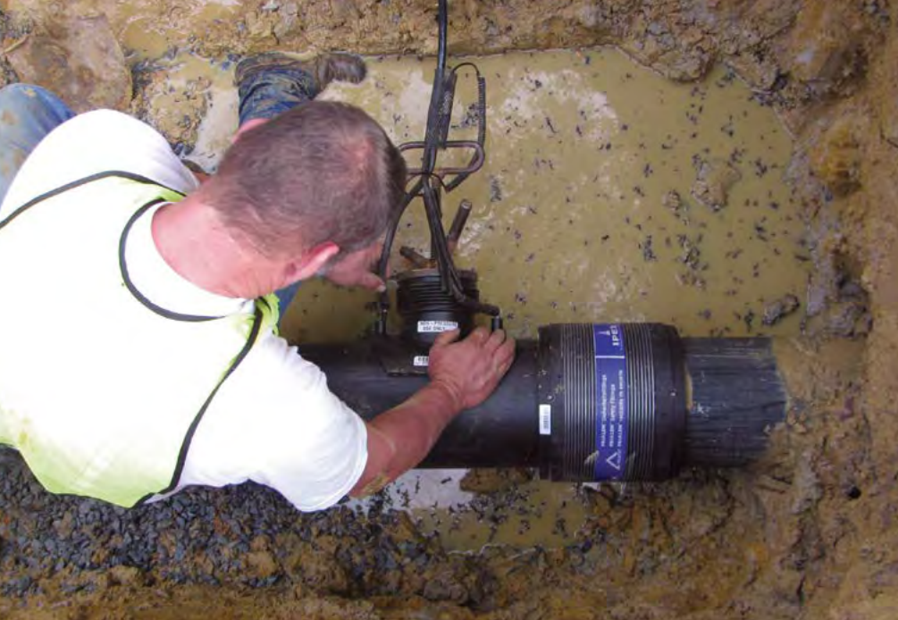
Installation of a fused-on gasketed lateral service fitting adjacent to an electrofusion coupling
