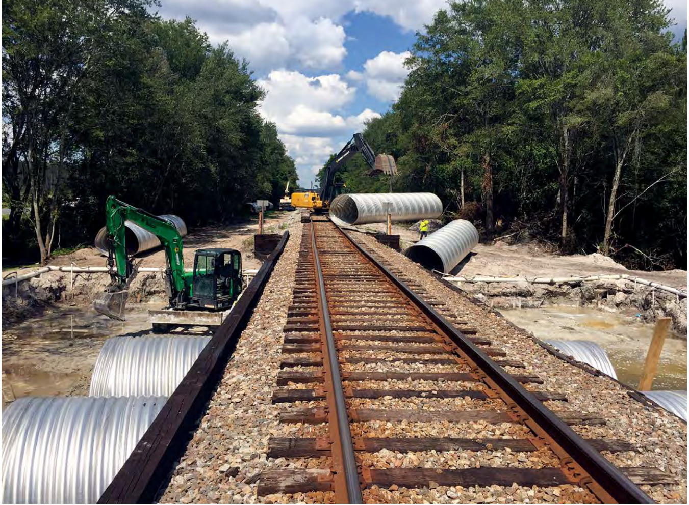
Most efficient cost-effective solution was sliplining with a multi-barrel corrugated steel pipe (CSP) culvert
