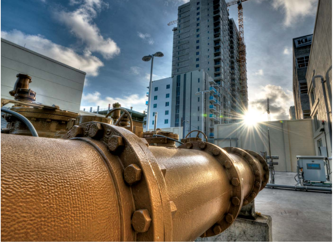
Pump station architecture and odor control were vital to meet Miami 21 zoning, due to location in the heart of downtown Miami
