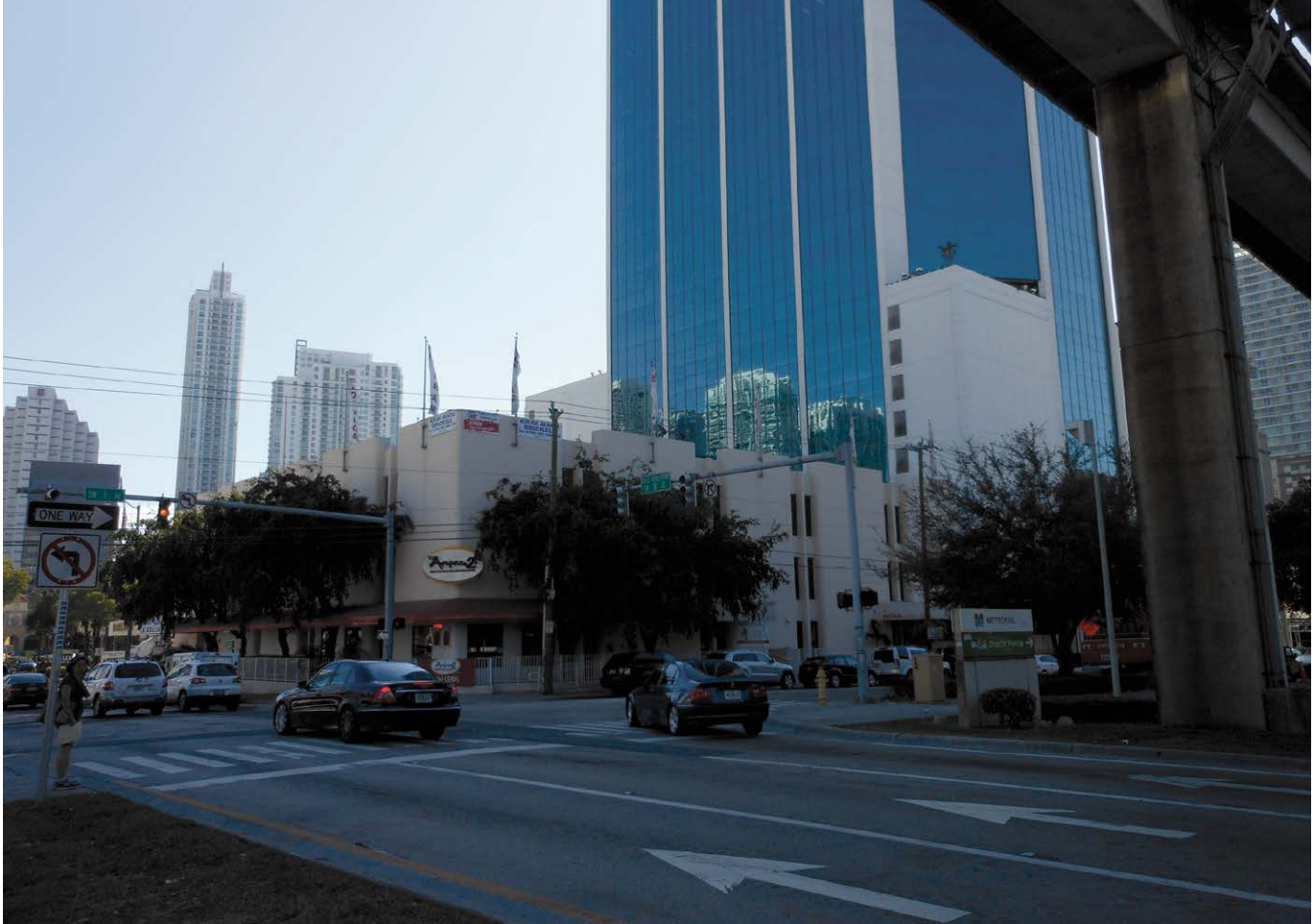
Foundation columns for an elevated rail line had to be navigated to install the receiving shaft in the heavily congested intersection of SW 8th Street and SW 1st Avenue
