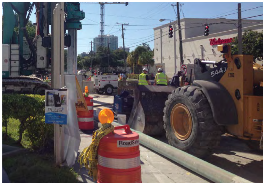
Existing overhead & underground utilities affected the routing of the new pipeline & choice of construction method
