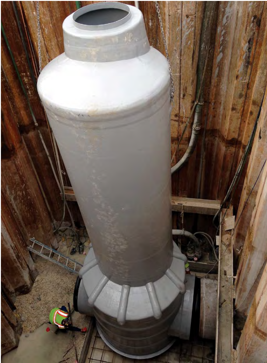
Shaft walls and floors were required to be designed to prevent movement caused by the combination of hydrostatic and ground forces, control upwelling of groundwater, and limit infiltration of groundwater into the shaft
