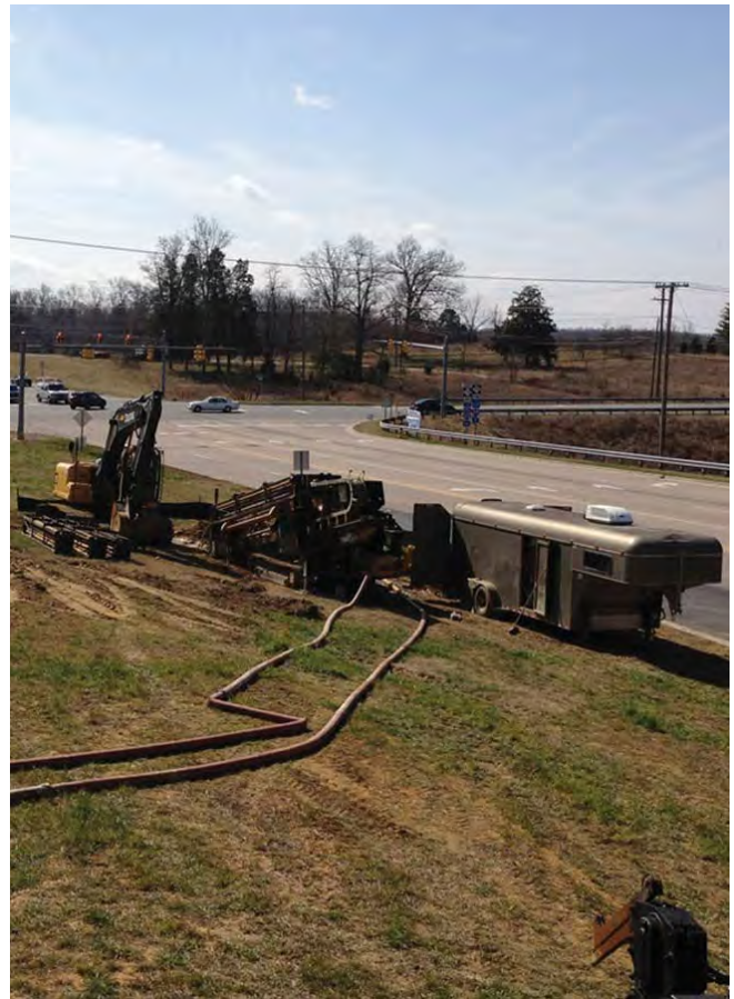
Delta has earned a solid reputation for successful HDD crossings and precise work in variety of challenging conditions
