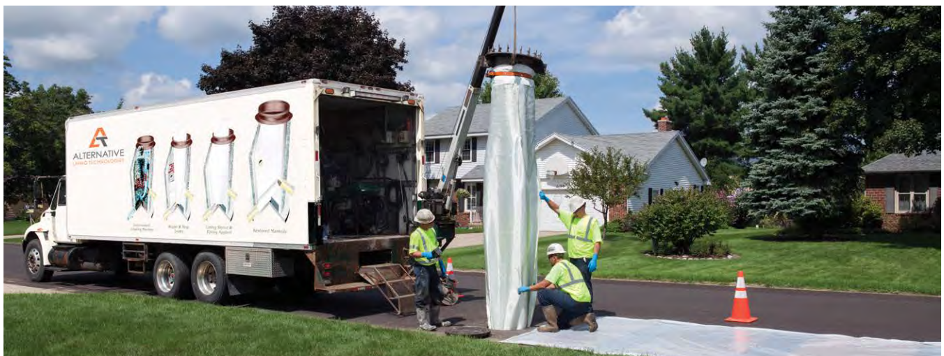
Epoxy resin is mixed and applied on site, then liner inserted into the manhole interior
