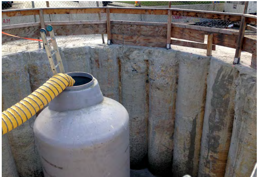
The secant pile shaft, at the busy intersection of SW 11th St and SW 2nd Ave, was the main launch shaft for three of the five microtunnel drives
