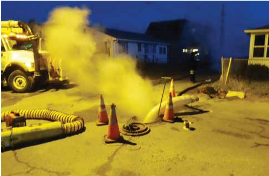
Lining & curing pipe into the night. The neighbors could not have been more hospitable
