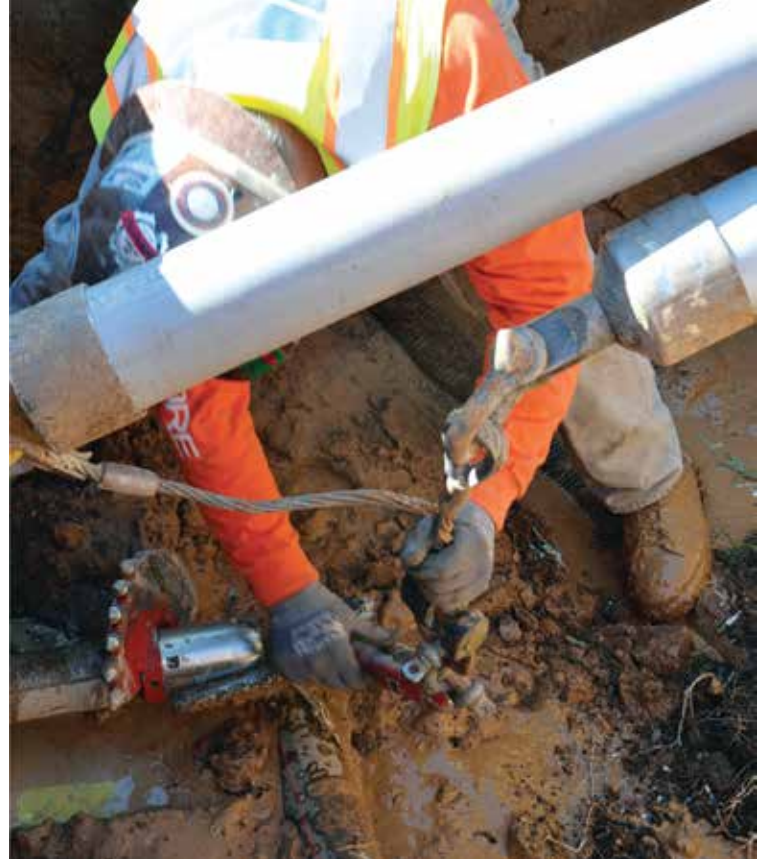
Attaching cable and product to the swivel in preparation for a direct pullback with the FastBack System. The cutter on the FastReam housing will enlarge the bore to pull multiple pipe
