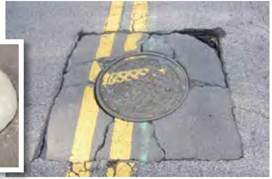
Many concrete pads can fail prematurely and disrupt traffic
