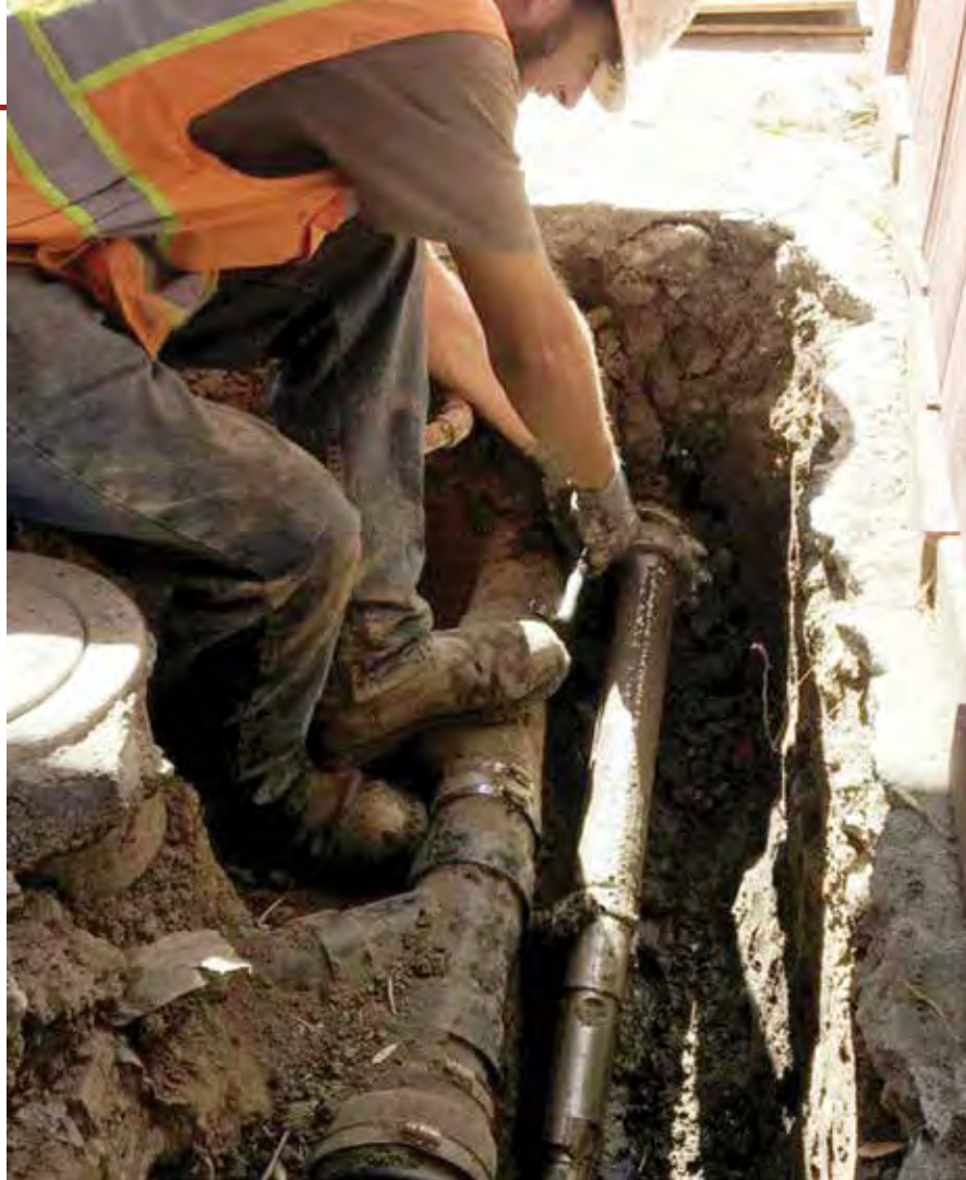
An example of the FastBack System boring close to existing utilities as well as in tight, closed-in conditions. In this instance it was a fiber installation next to a sewer main and a fence. The driller was able to pull his utilities without removing any structures or disrupting any existing utilities
