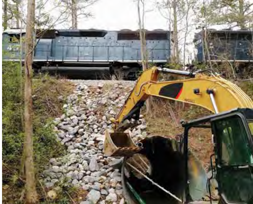
AGR preferred a method that would allow the railroad to remain in operation while construction took place
