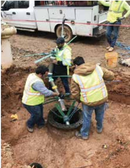
Insertion of PipeDiver in 24-inch Manway
