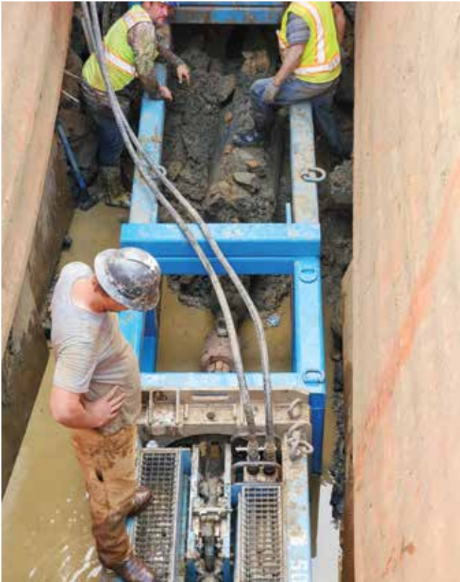
H&H Site Specialty utilized a Grundoburst 1250G static bursting unit from TT Technologies. The challenging burst took place under a 4-lane interstate where no digging was allowed
