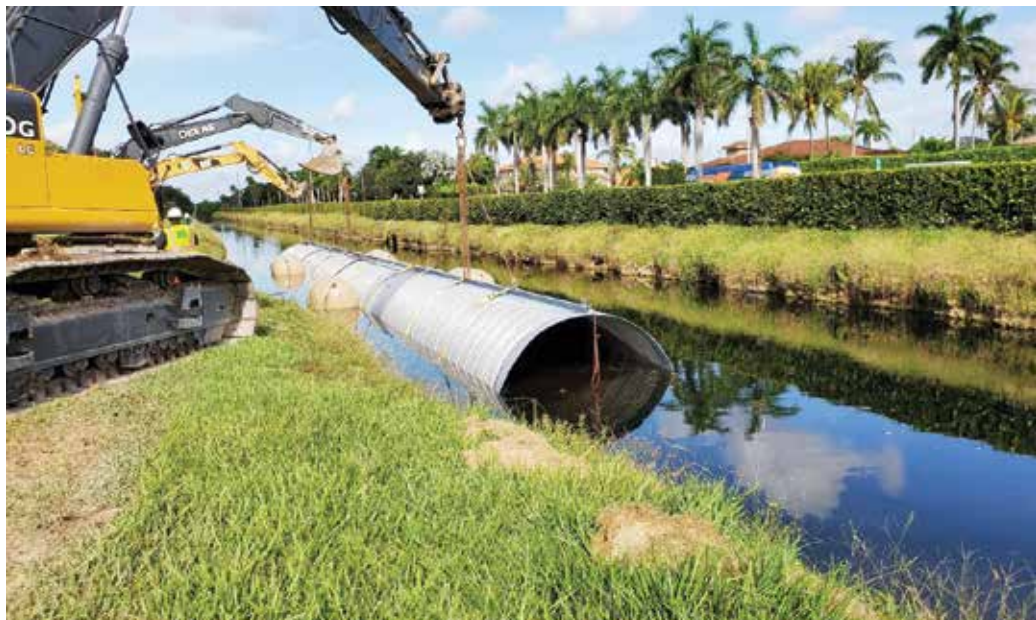
The liner pipe was installed under live flow using a unique anti-buoyancy method
