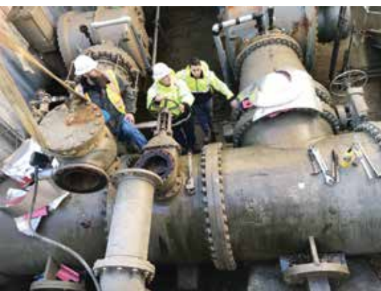
SmartBall Insertion in 12-inch Surge Valve
