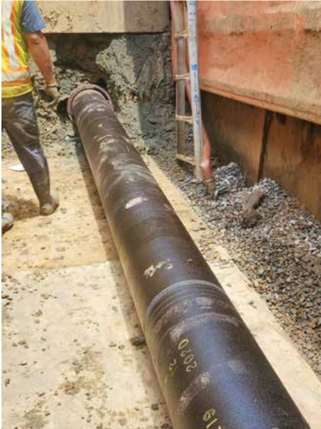
Static pipe bursting systems are able to install a wide range of product pipe. For the burst under I-675, H&H Site Specialty burst the existing 8-inch ductile iron and replaced it with 12-inch ductile iron.
