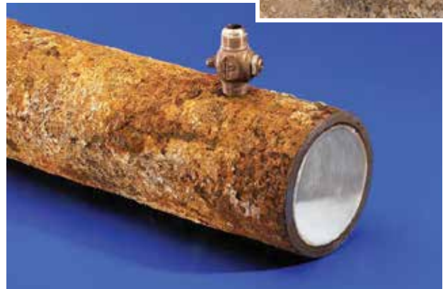
Figure 1. Examples of Deteriorated Pipelines
