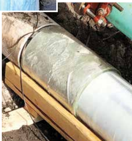
Figure 4. End termination of a 10-inch Force Main in Central Florida
