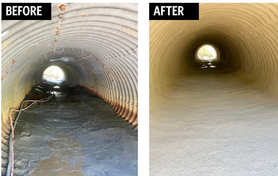
Figure 5. Structural rehabilitation of twin 74-inch X 96-inch Arch Plate CMPs – an entirely new pipe built inside of the old pipe
