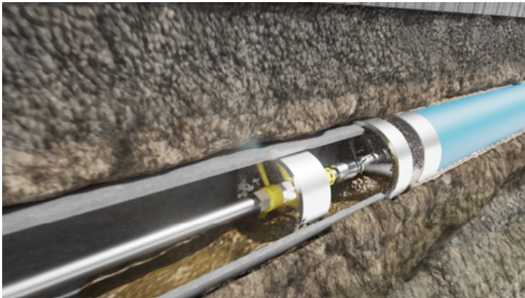
Figure 3. Grinding of AC pipe and mixture with drill mud creates the slurrification during the process
