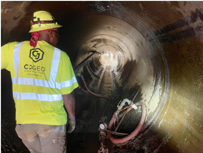
The second lift of grout was pumped through the longest sacrificial pipe
