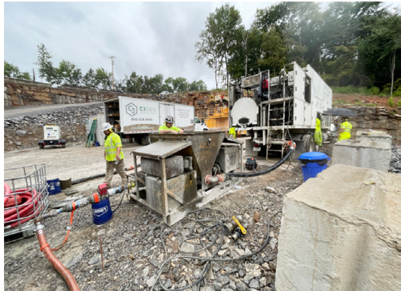
The annular space grouting was completed in just over two days in two lifts
