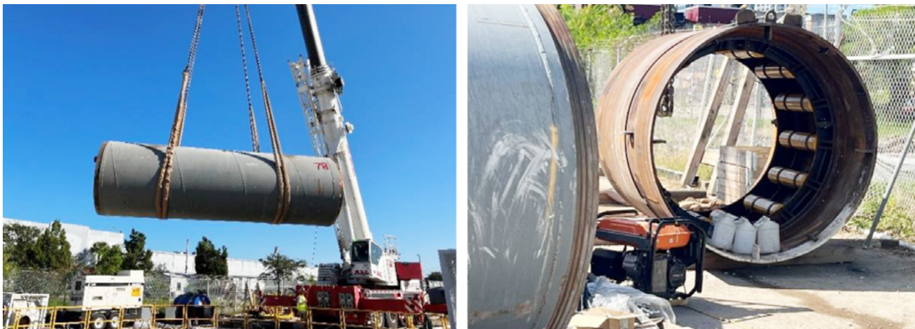
Figure 7: Tri-Loc pipe joint being lowered into shaft (left) and Intermediate Jacking Station being built out (right)
