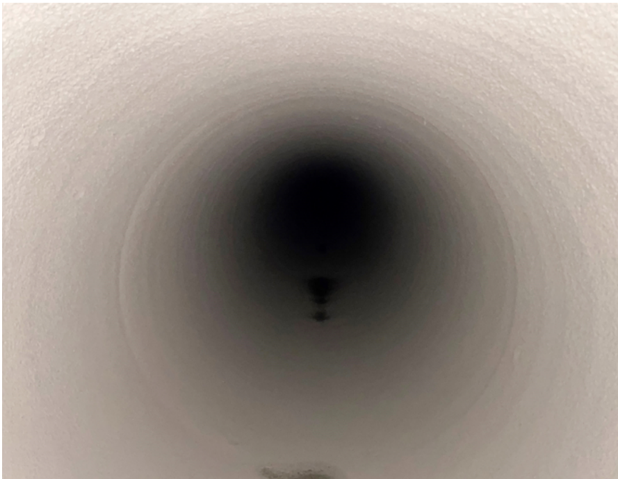
Figure 8. More than 30,000 LF of pipe culverts of varying sizes have been structurally rehabilitated using geopolymer SAPL
