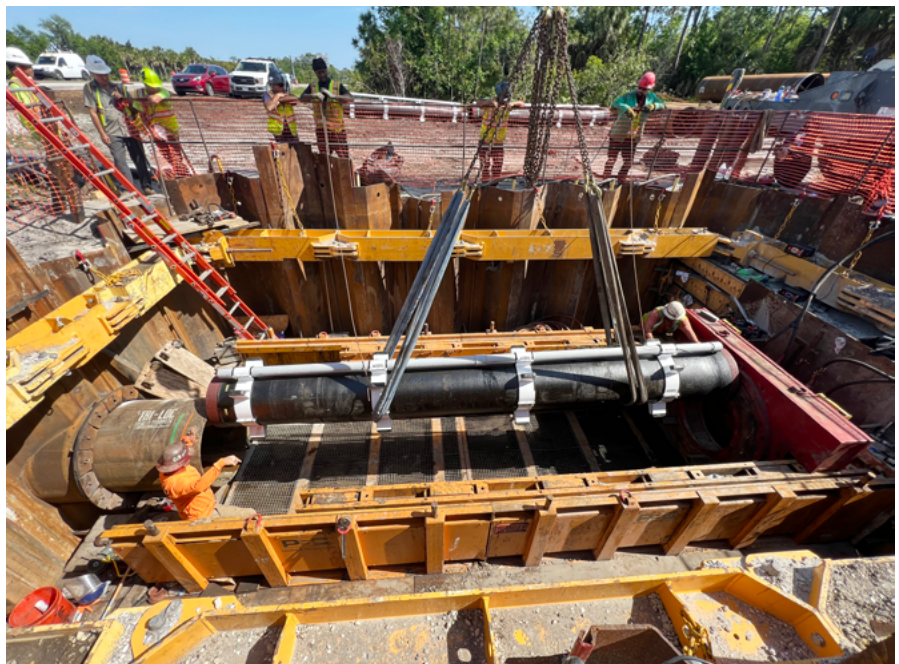
Carrier pipes included 24-inch DIP and 4-inch PVC conduit for a fiber optic line
