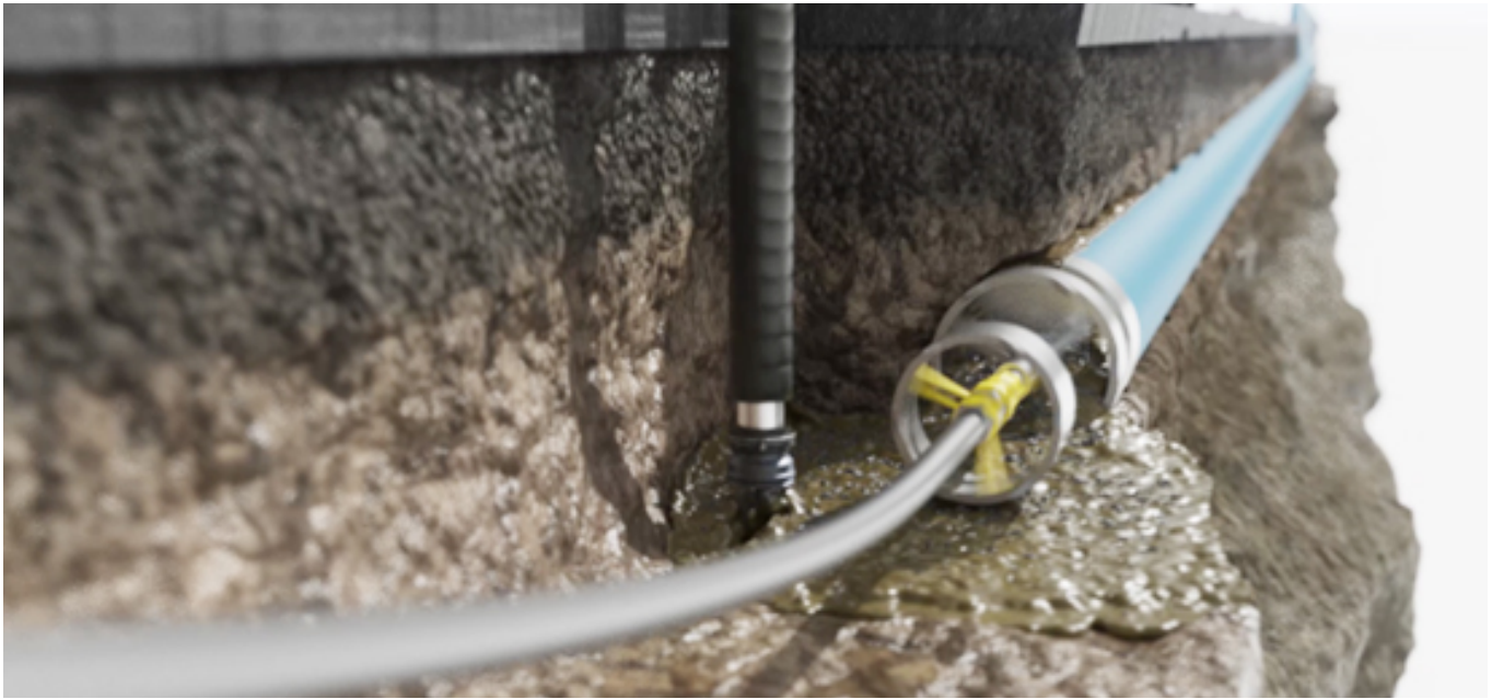
Figure 5. The slurry mix is vacuum excavated from the access pit and hauled away for disposal
