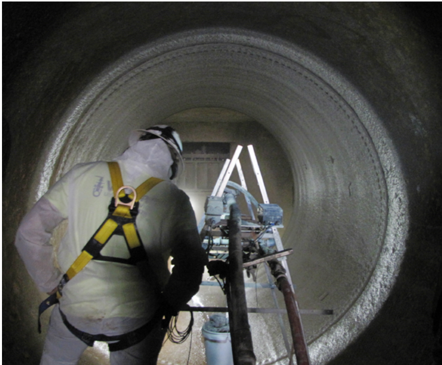
Figure 7. Geopolymer is often applied by spin casting in large diameter sanitary and combined sewers, manholes, wet wells and other related structures
